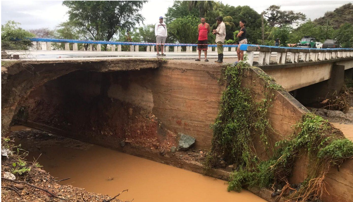
Bridge washed away in Santiago de Cuba province (Source: TVSantiago )
